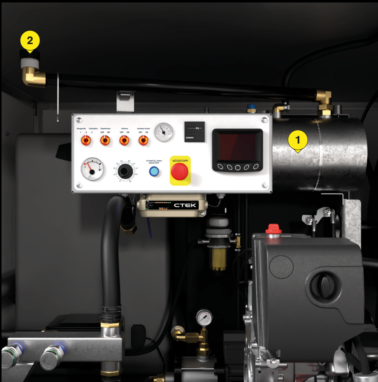
1 Expansion tank with level tube
